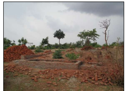
A permanent church building is being constructed under the godly leadership of Pastor Benson.
